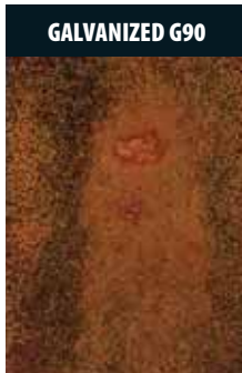
After 23 years of exposure, this hot-dipped galvanized G90 test panel exhibits almost complete red rust.
